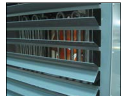
Detalle deflectores. View of deflectors.
